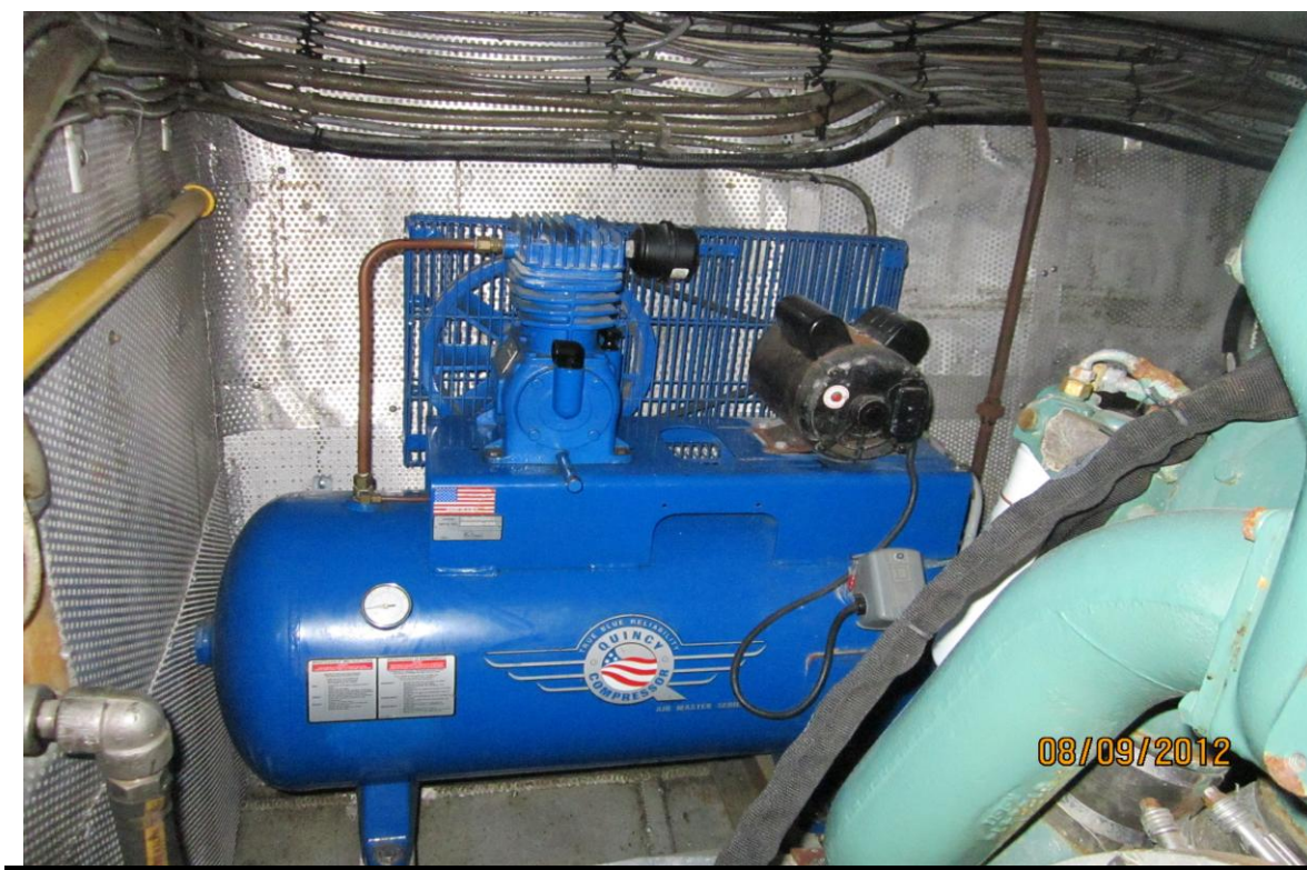
Photo 14, Air compressor located fwd. stbd. side engine room.
