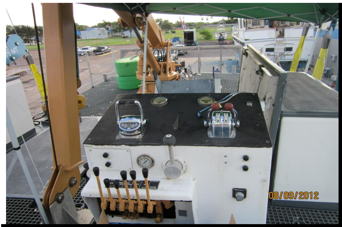
Photo 8, Aft control station.
