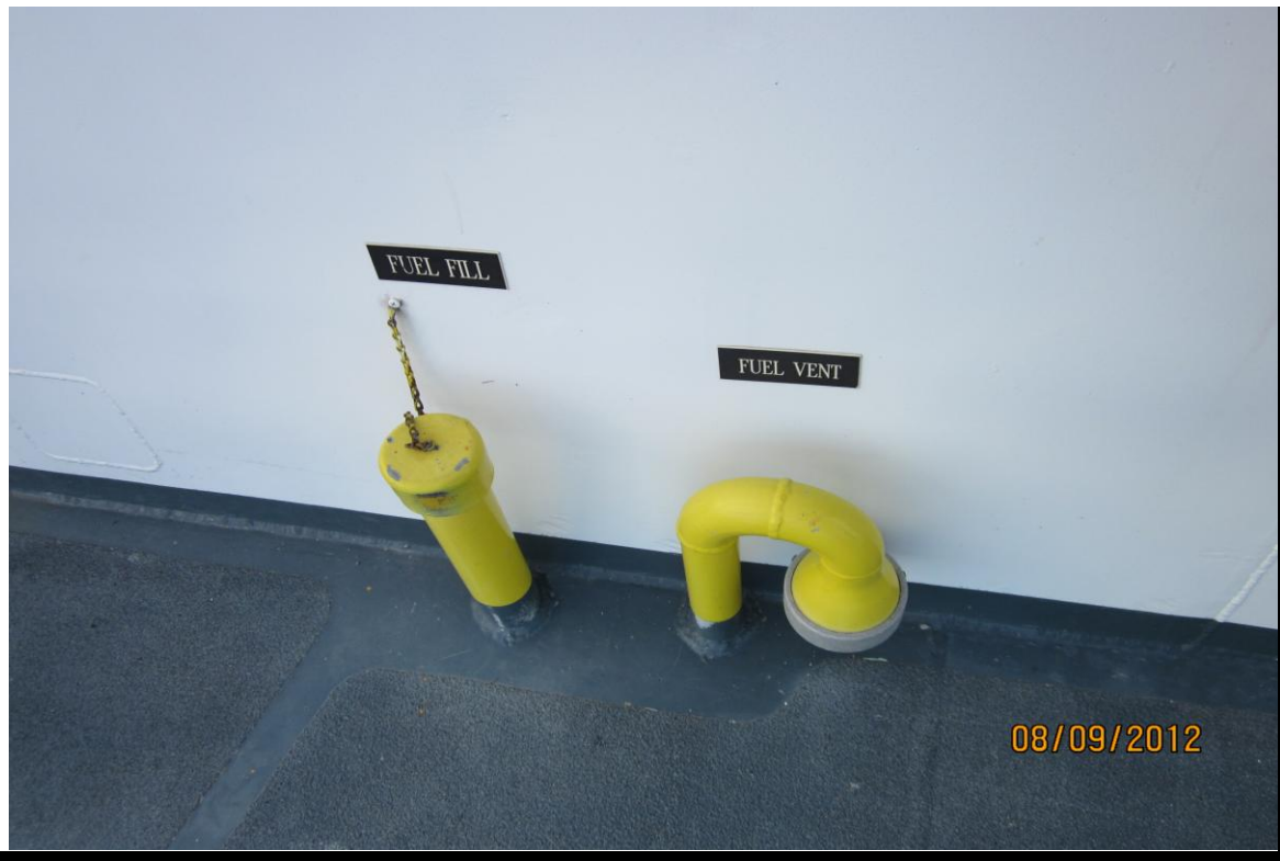
Photo 9, Stbd. side fuel fittings. Same on port side.
