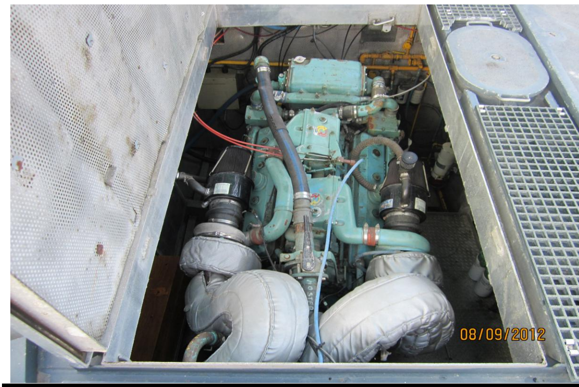
Photo 13, Port engine seen from deck. Note heavy insulation installed. Stbd. side same.
