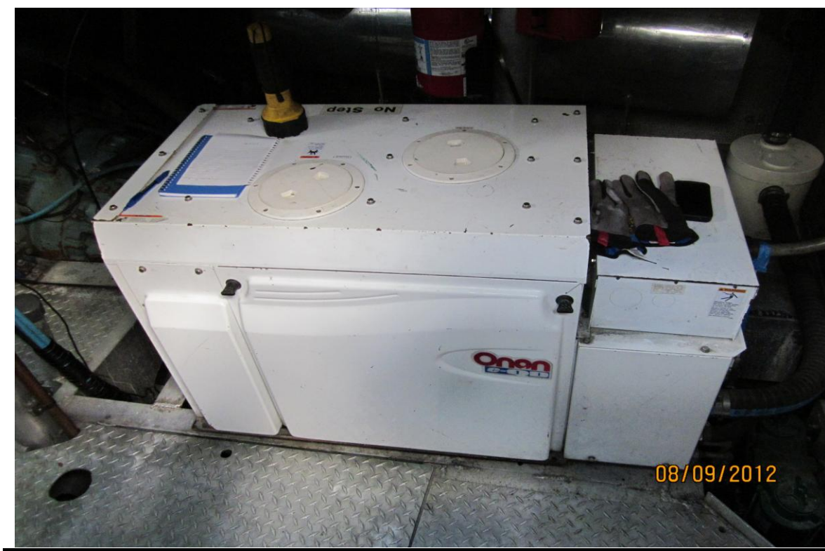
Photo 15, Onan Generator set, aft engine room.
