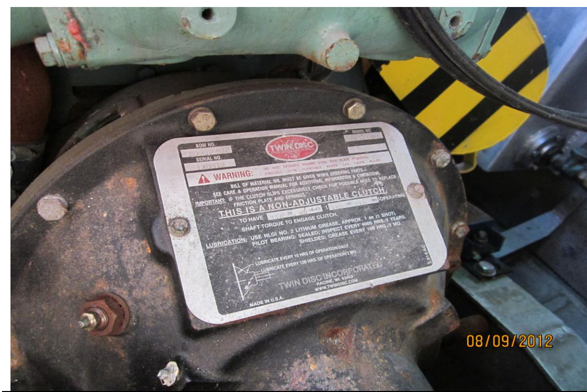
Photo 16, PTO in front of port side engine driving crane hydraulic system.
