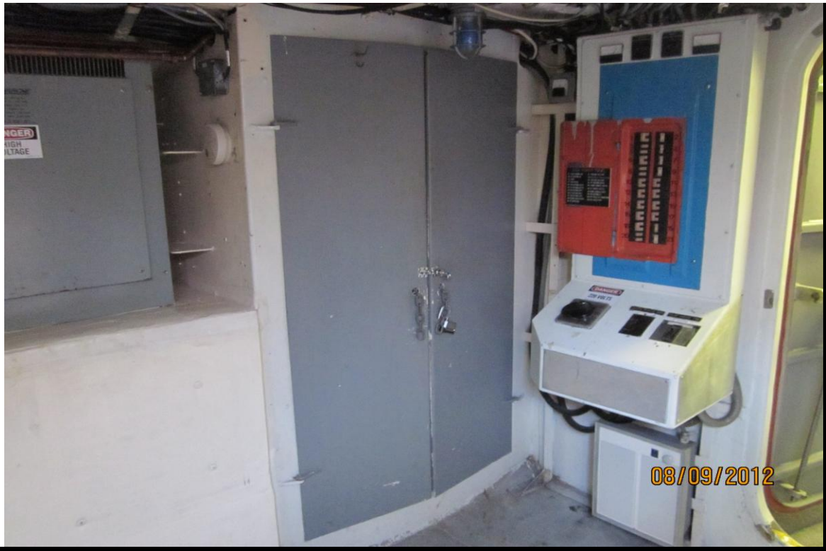
Photo 18, Work room just aft of sleeping quarters with primary electrical panel.
